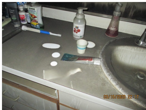
Figure 4: Adhered fire residues
