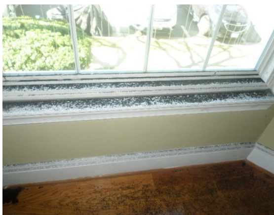
Figure 3: Non-adhered Fire residues
