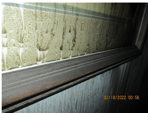
15 16 Figure 5: Condensation streaks on glass
