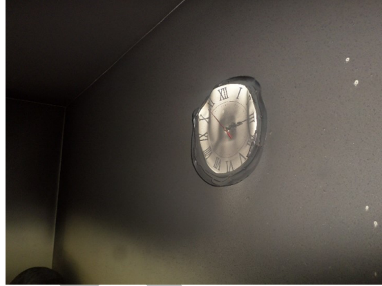
Figure 2: Heat damaged contents above heat line
